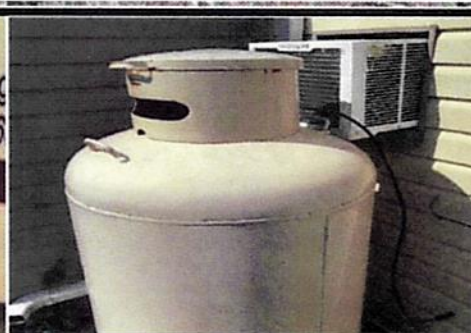
This could be a DOT or ASME tank. This tank should not be located closer than 5ft from any air intake.
