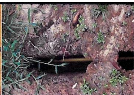
This line was barely covered and exposed to harmful UV rays from the sun.
