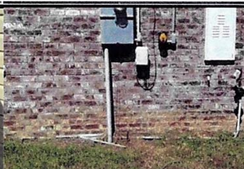
This regulator is too close to an ignition source. It should be 5ft away.
