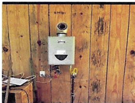
This is an indoor hot water heater installed under a porch. This should be an outdoor unit.
