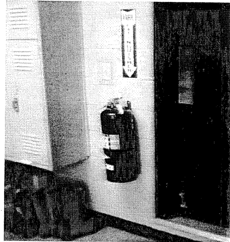
Figure 1. Fire Extinguisher Station
